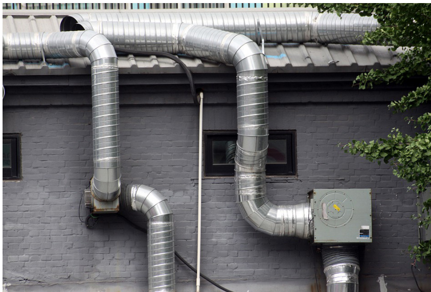
Figure 2. Examples of poor integration of the ventilation system with the building.
