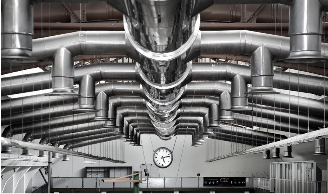
Figure 17. Different degrees of architectural integration of the ventilation system.
